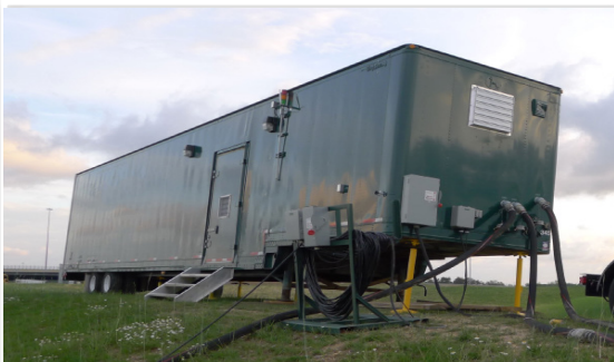
Suspended solids removal system
