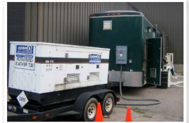
Dual phase extraction system trailer (DPE)
