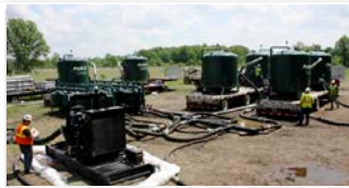
Above: 1500 gallon per minute water treatment
